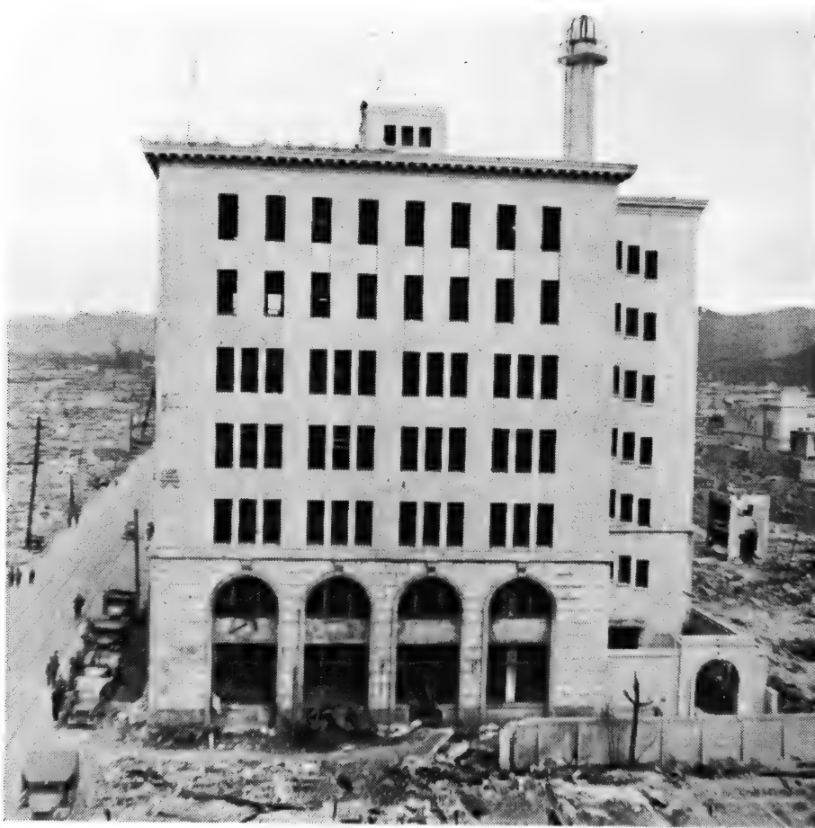
Photo No. 7. HIROSHIMA. Reinforced concrete building about 300 yds. from the centre of damage, which is to the left of the photograph. There was no serious structural damage, although a roof panel was depressed and some internal party walls were deflected. Designed for earthquake resistance, this building has a composite reinforced concrete and steel frame. See paragraph 24.
